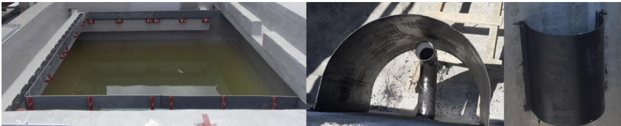
Figure 3. A combined photo of existed settling tank with dimensions 5 m Length * 5 m Width * 4 m Height and two views of installed diffusion drum
